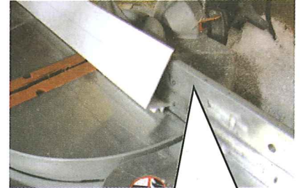
Cut a straight cut on your chop saw so the clad butts up to the header jamb cover. Make sure to cut the correct end so the sill angle will match on the bottom.
